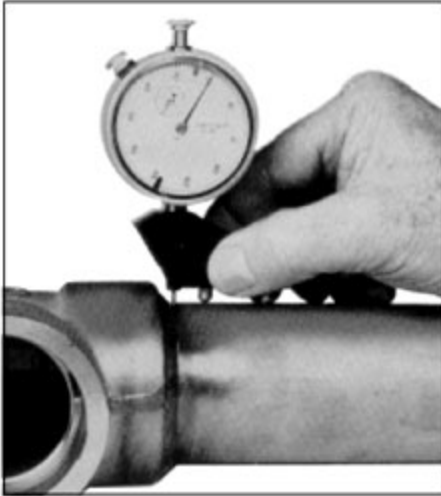
Measures Undercut Socket Weld
